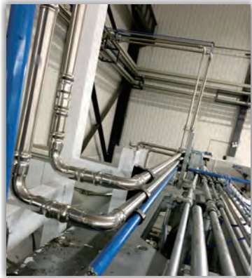
● Cooling water for Auto Parts.
