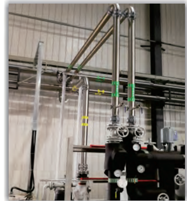
● Oil and Cooling water for Machinery.
